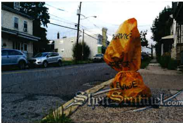
Photo 1. Inoperable fire hydrant bagged by Aqua until replaced. Shensentinel newspaper, August 10, 2023.
