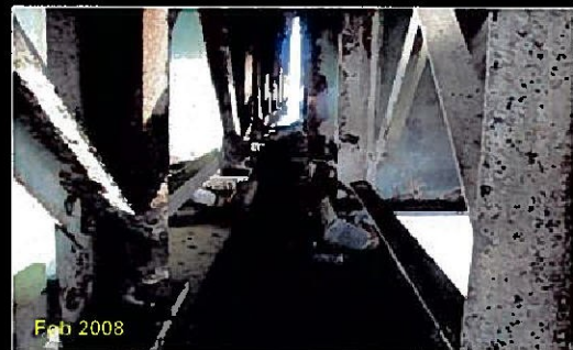
Birmingham Bridge Tipped over Rocker Bearings at Pier 10S Allegheny County
