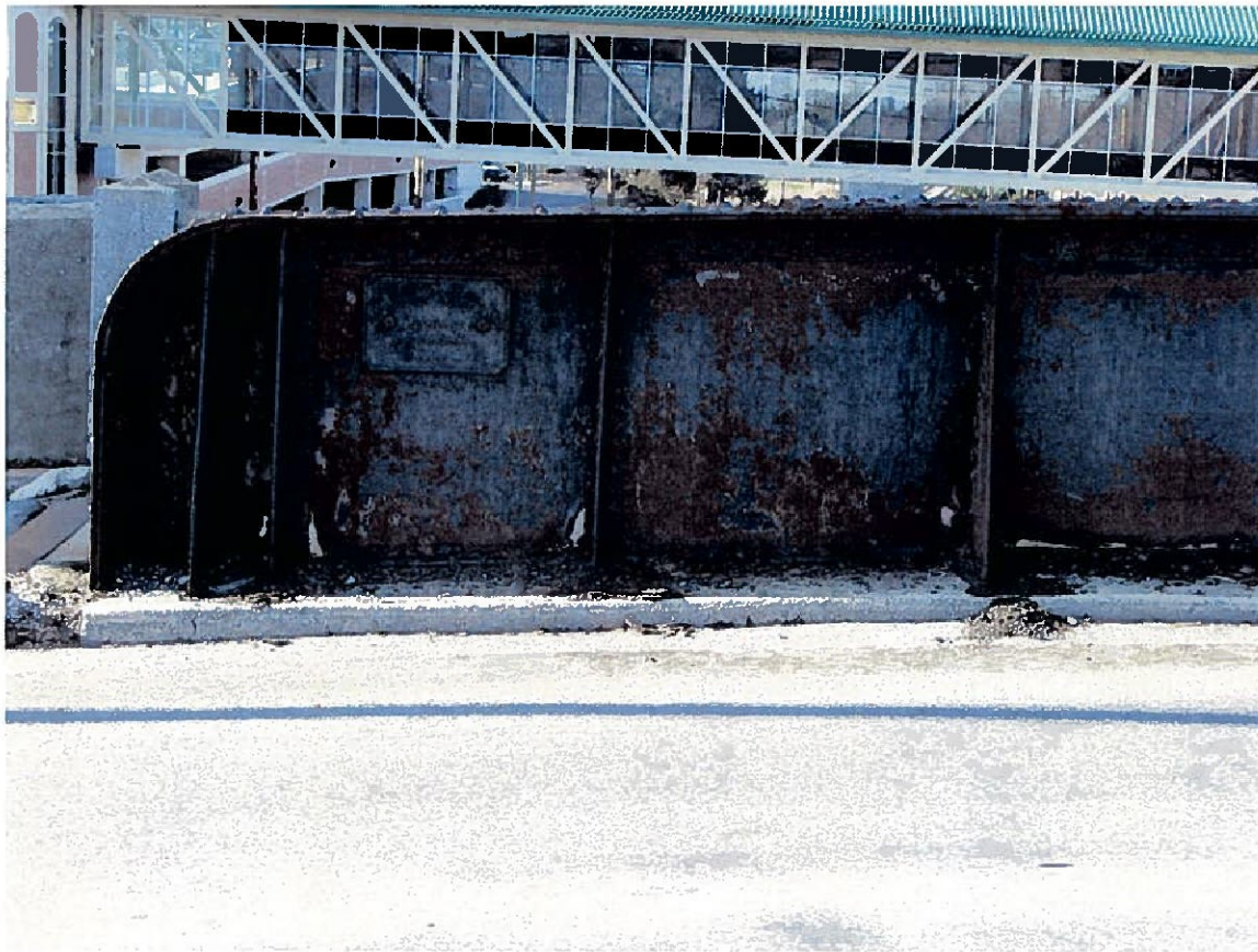
Web deterioration on SR 743 in Hershey – January 2008
