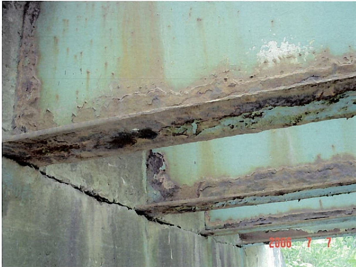
Bottom flange section loss and rusting of webs near backwall in Somerset County (SR 2037)
